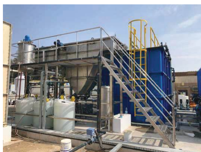
Effluent Treatment Plant
