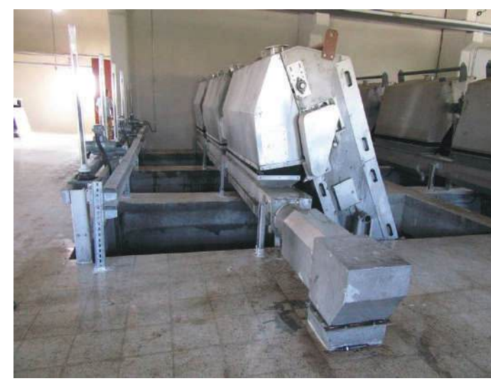
Screw Conveyor & Compactor
