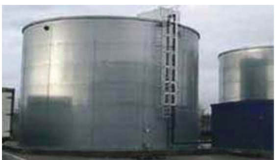
Fire & Potable Water Tanks
