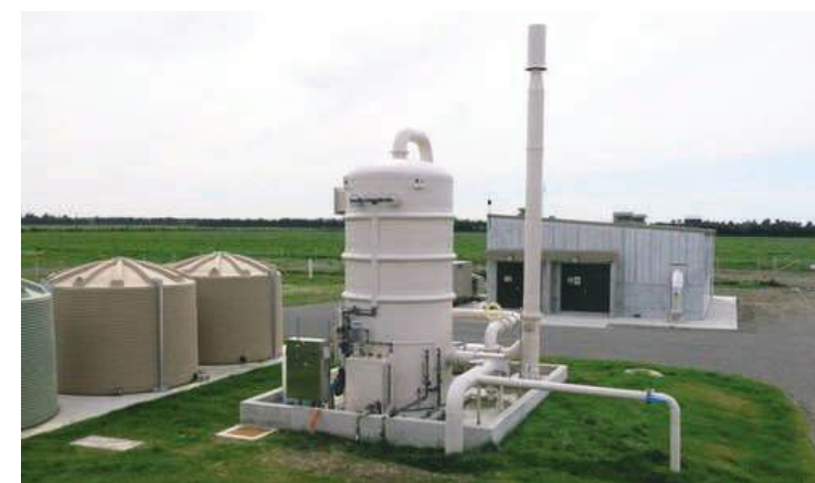
Odor Control Unit
