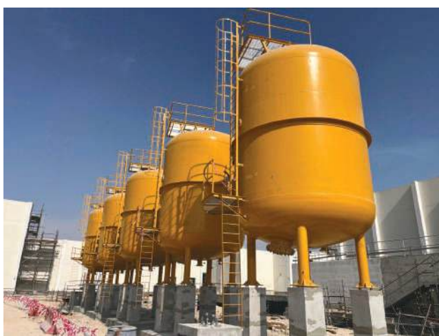
Multi Media Filtration System
