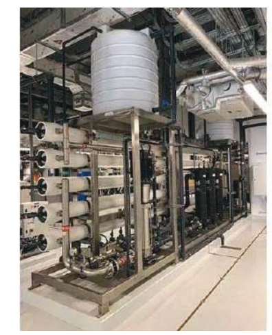
Effluent Treatment Plant
