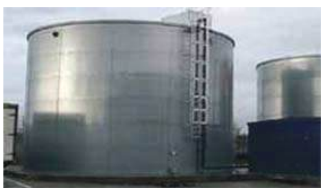
Fire Water Tanks
