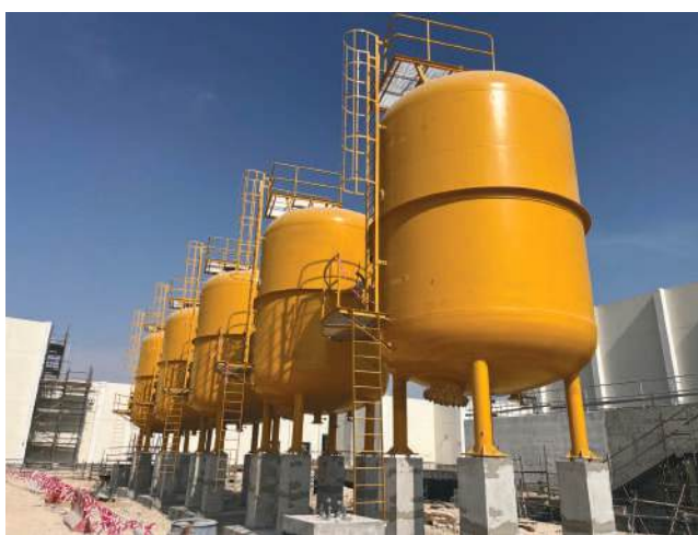
Multi Media Filtration System
