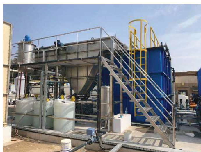
Effluent Treatment Plant
