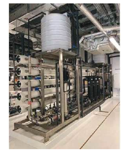
Effluent Treatment Plant
