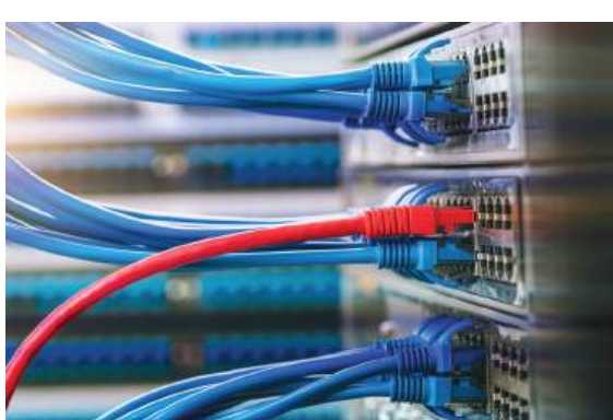
Structured Cabling System
