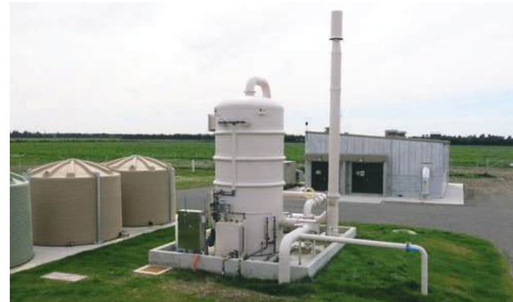
Odor Control Unit
