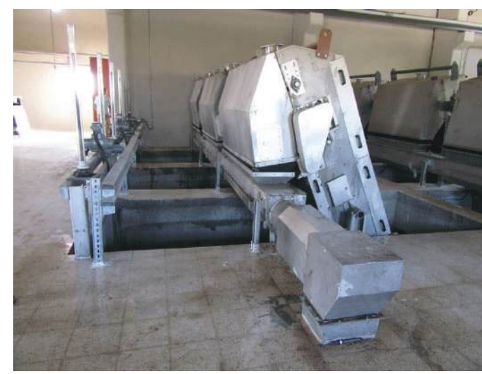
Screw Conveyor & Compactor
