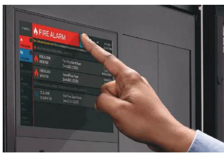
Fire Alarm & Air Aspiration System
